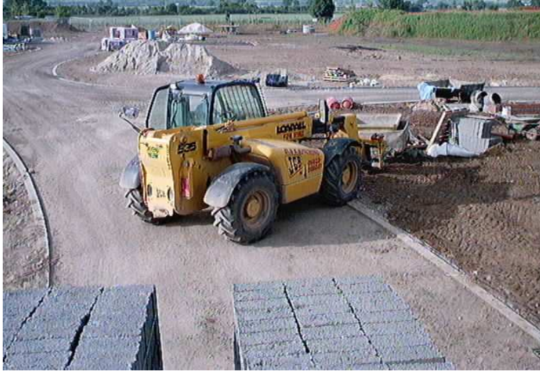
An all-wheel-drive fork truck may prove to be worth its weight in gold on a busy site!
